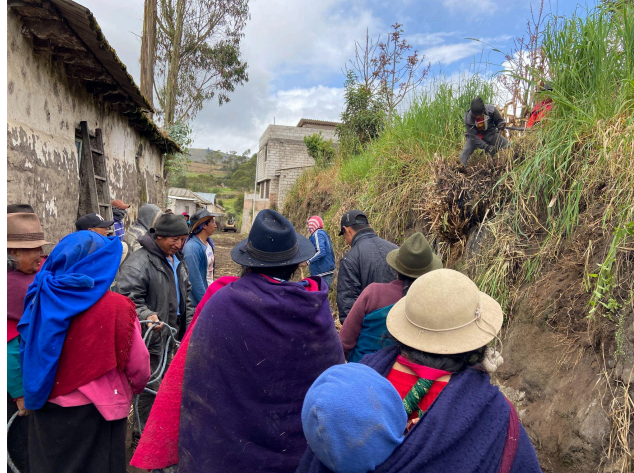
Elderly community members, mothers' carrying children, and the few young people of Caliata working vigorously at removing debris from the blocked waterway.
